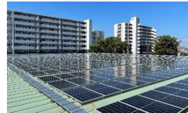
Solar panels on top of LIVRE KEISEI Albis Maebara
