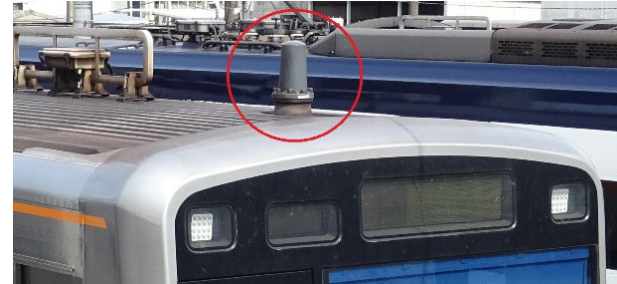
Antenna installed on train roof
