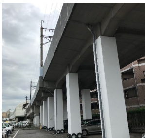
Track elevated for better earthquake resilience (between Chiba Chuo Station and Chibadera Station)
