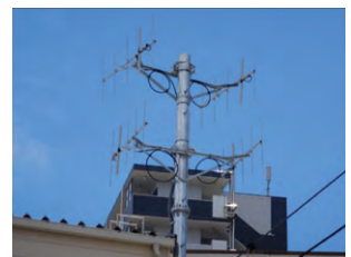
Ground base station antenna
