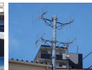
Ground base station antenna
